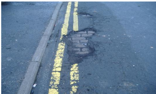
Surfacing failure caused by underlying setts
