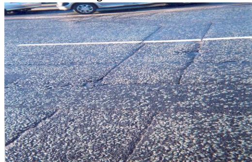
Cracking from utility trench
