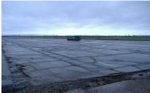
Reflective cracking from concrete bays
