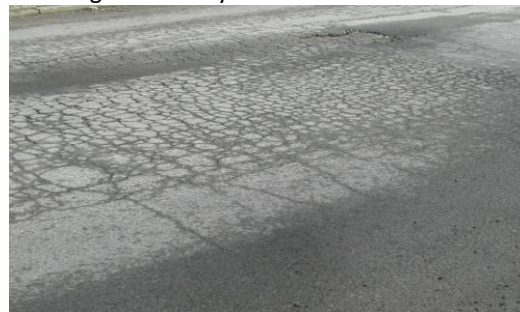
Alligator cracking due to structural failure
