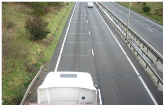
Reflective cracking from expansion joints
