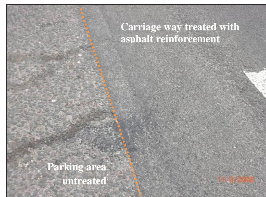
Close up area showing prevention of cracking
