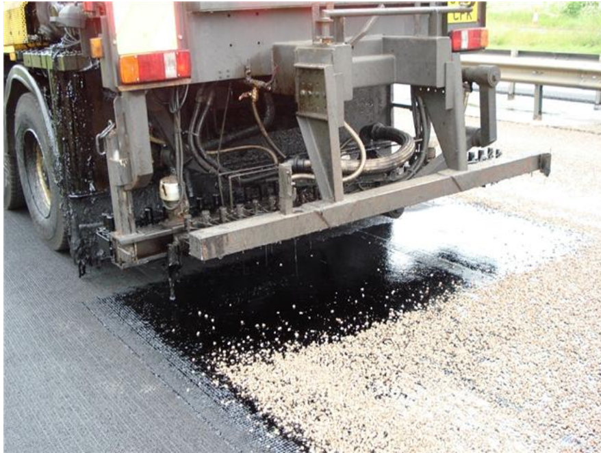
Protective layer of chippings applied onto a PMB sprayed on a Geosynthetic
