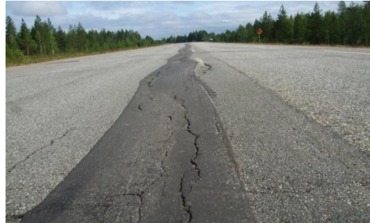
Reflective cracking from thermal movement
