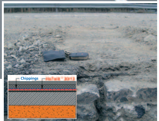
Part of German Highway 13 broken out during reconstruction in 2005 – remaining asphalt binder course above HaTelit® – no visible cracks
